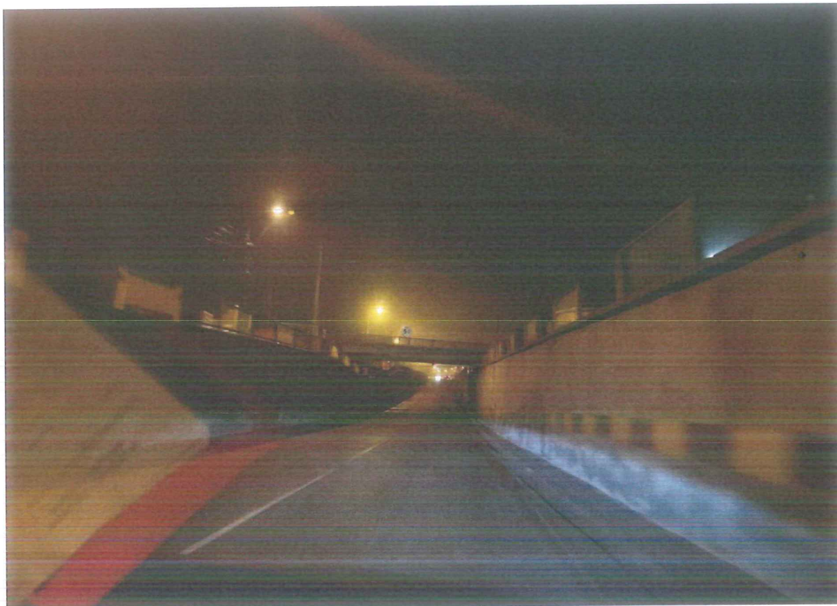
Tunel zona lidll drum European iluminat necorespunzator-fenomen de
